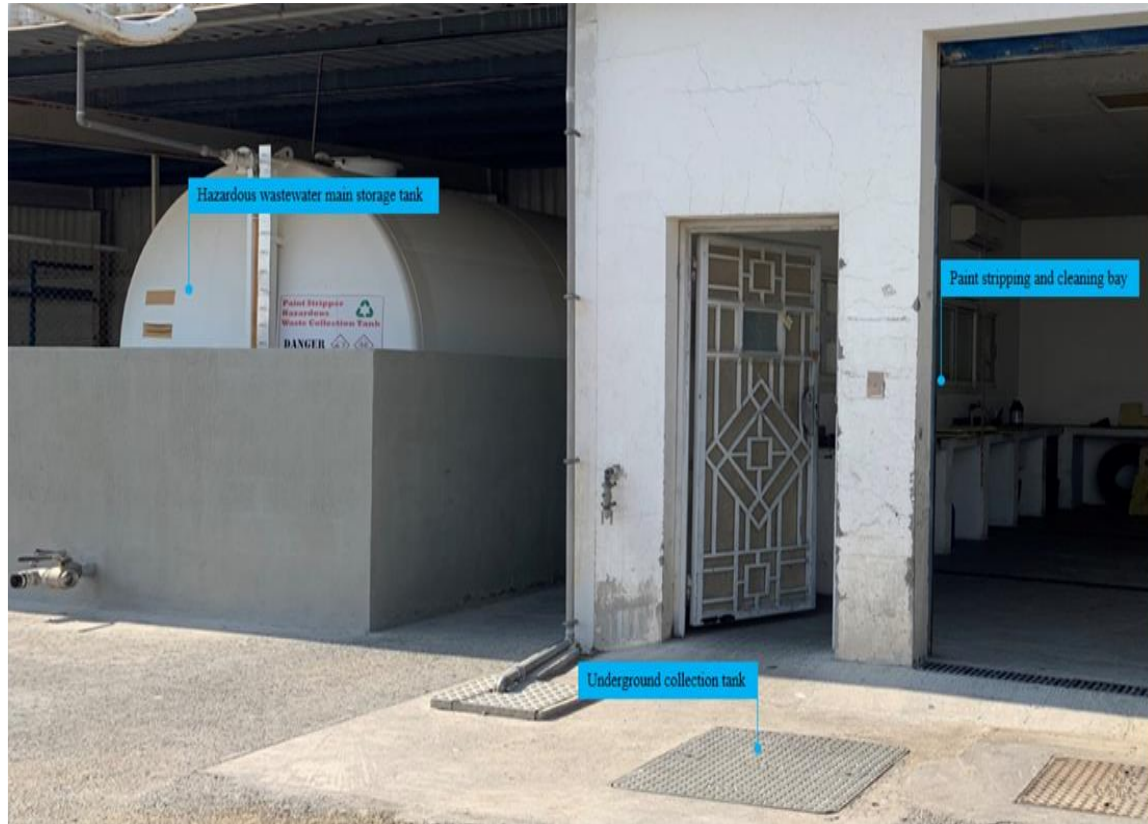
Paint stripping and cleaning facility
